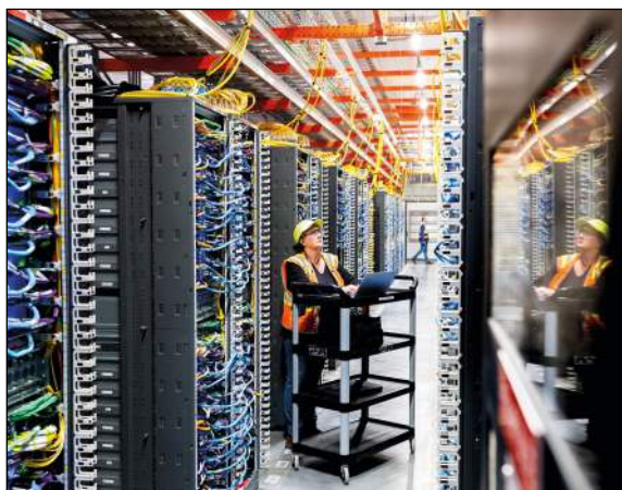
An Amazon Web Services data centre in New Carlisle, Indiana
